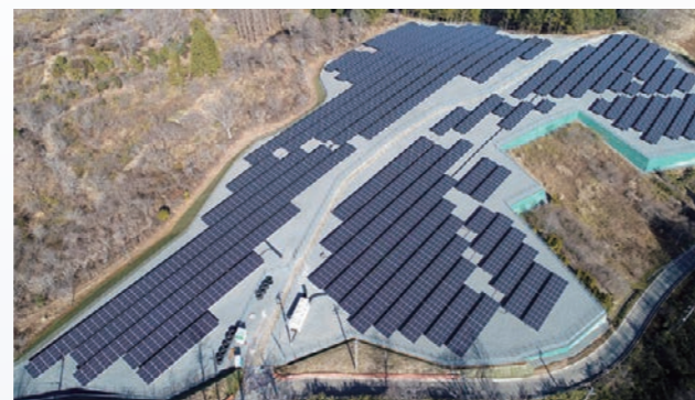
Tochigi Motegi Solar Park (SB Energy Corp.)
