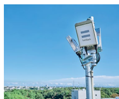
Base station antennas
